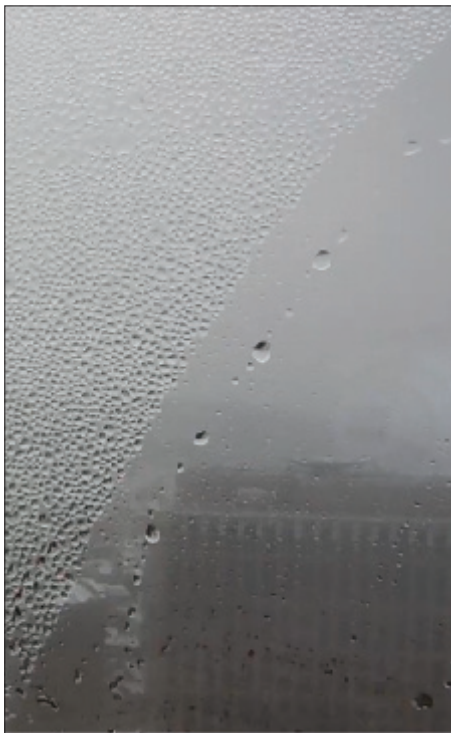
Figure 28 Condensation on a Window Source: Australian Glass and Window Association
